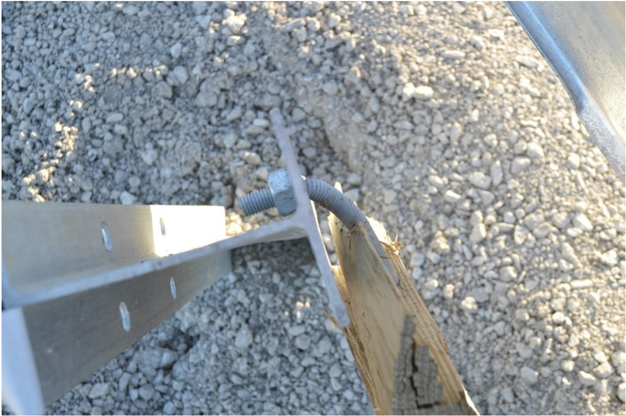
Figure 56. Bolt Damage. Test No. MGS7S-2
