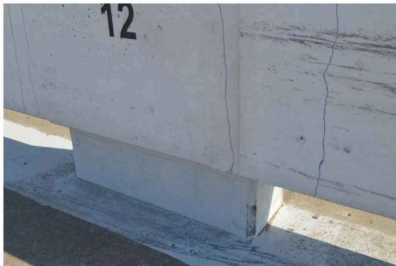
Figure 54. Concrete Post Damage, Post Nos. 11 and 12, Test No. OCBR-1
