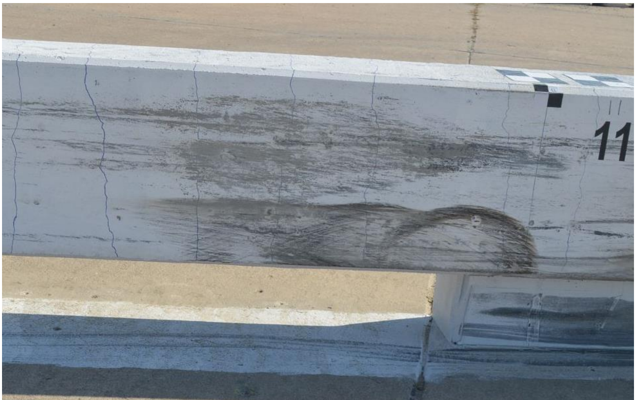
Figure 53. Concrete Beam Damage near Post No. 11, Test No. OCBR-1
