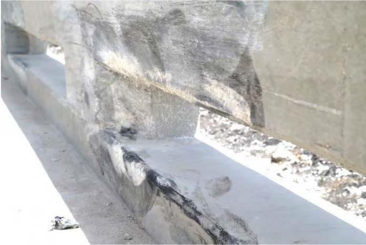
Figure 21. Lateral Extent of 2270P Vehicle Tire Marks on the T224 Bridge Rail [2]
