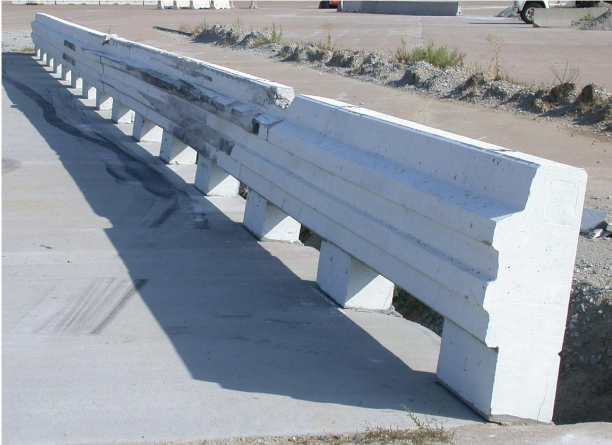
Figure 24. NDOR TL-5 Aesthetic Rail Damage [21]
