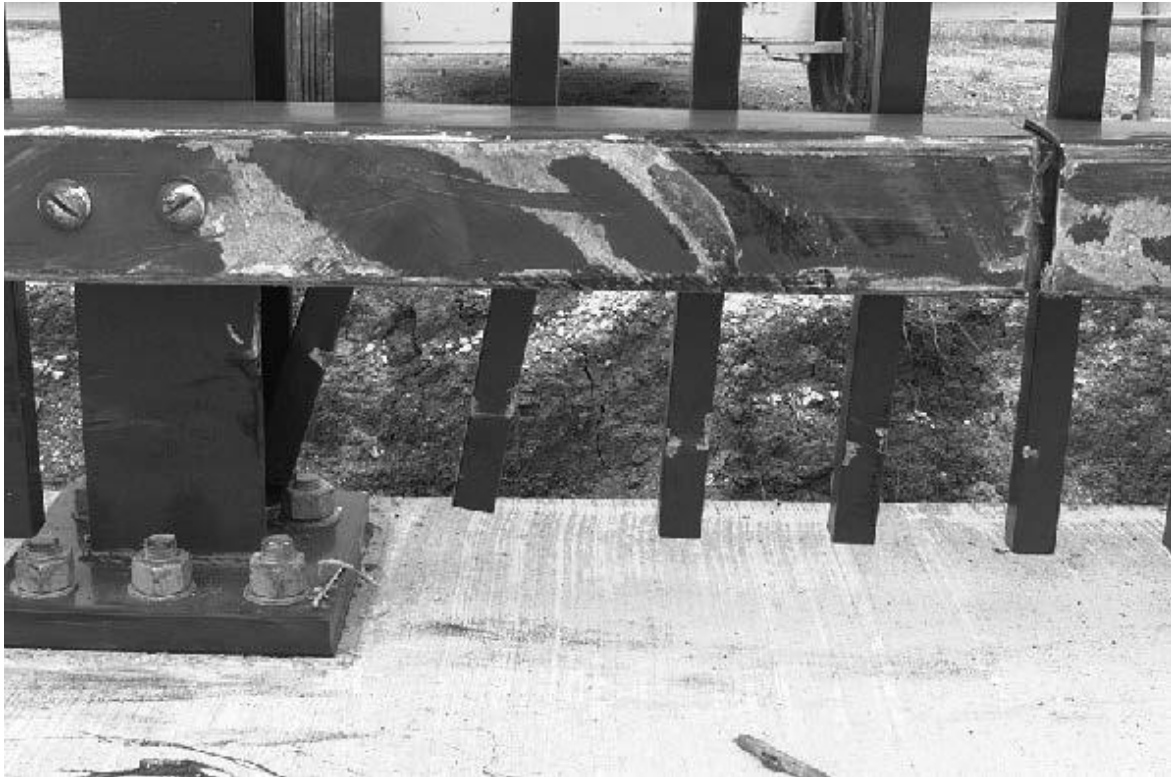
Figure 51. Lateral Extent of 2000P Vehicle on the Massachusetts Type S3 Bridge Rail [28]
