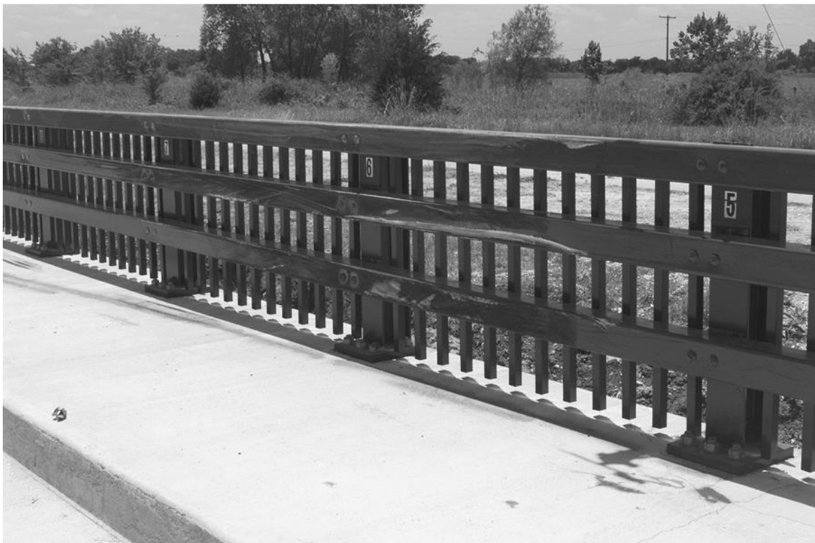
Figure 52. Lateral Extent of the 8000S Vehicle on the Massachusetts Type S3 Bridge Rail [28]
