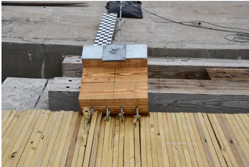
(a) Front View of Damaged Rail, Scupper Blocks, and Deck
