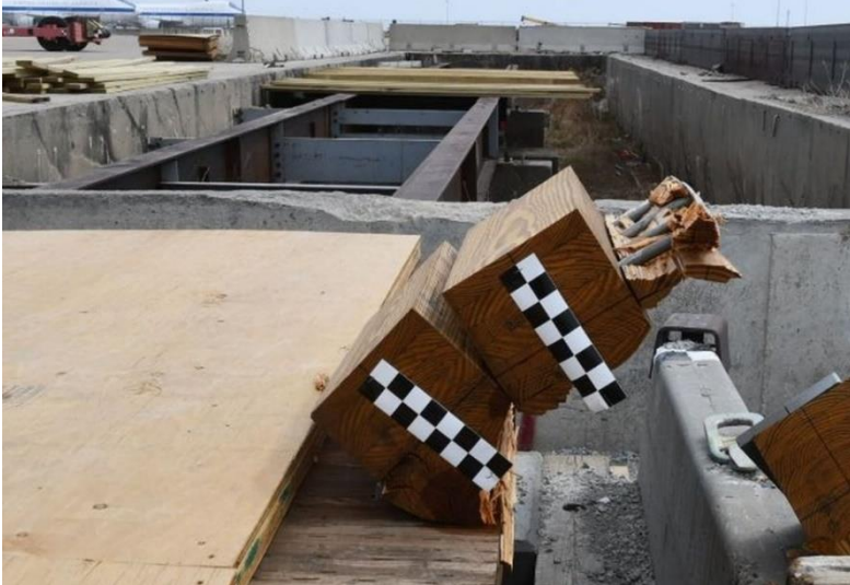
(c) Right-End View of Damaged Rail and Scupper Blocks
