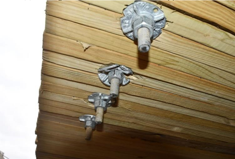
(b) Damage to Malleable Iron Washer and Deck
