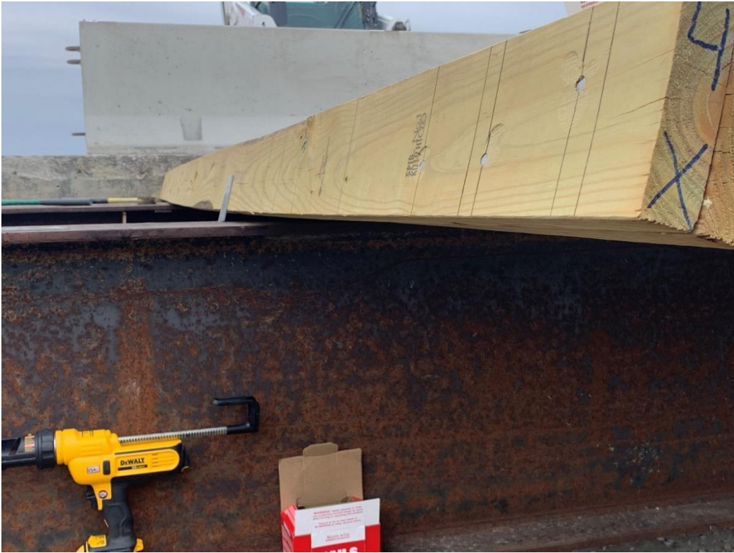
(b) Leaning of Boards on Nail-Laminated Deck
