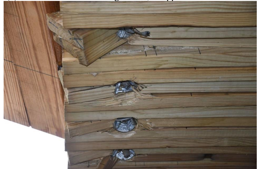
(d) Damage to Malleable Iron Washers and Deck
