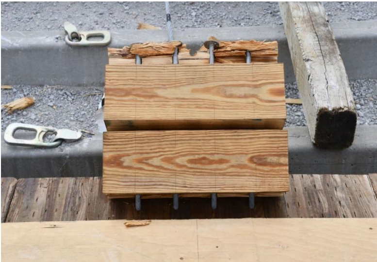
(a) Front View of Damaged Rail and Scupper Blocks
