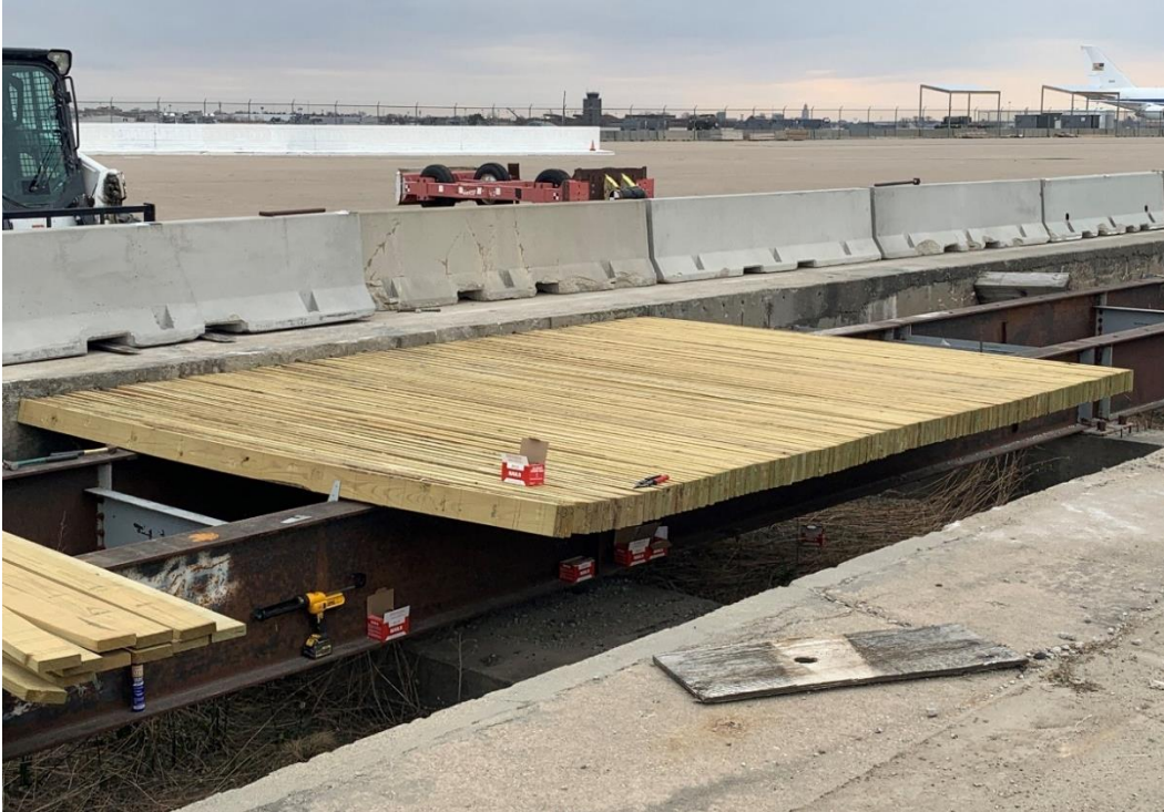
(a) Warping of Nail-Laminated Deck Off of the Girders
