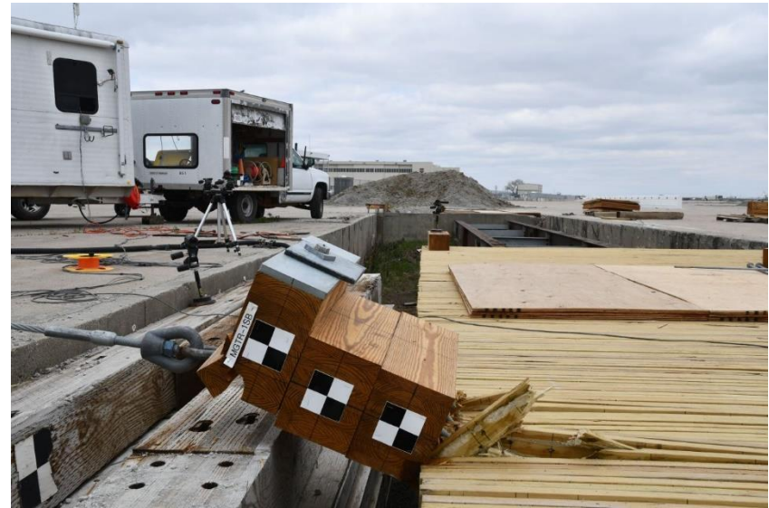
(b) Left-End View of Damaged Rail, Scupper Blocks and Deck
