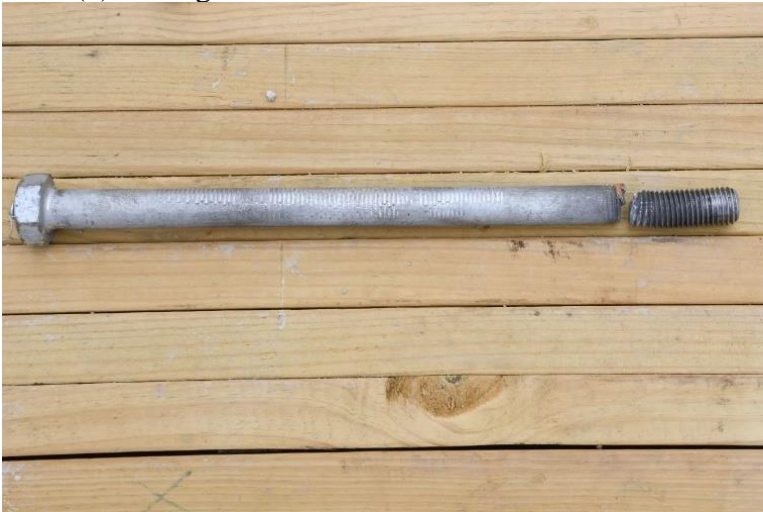
(c) Ruptured Bolt Used to Load Rail and Scupper Blocks
