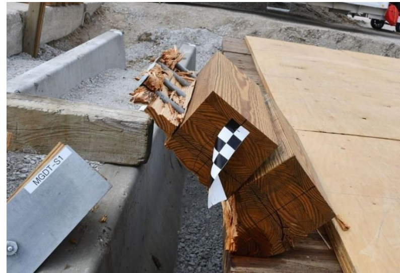
(b) Left-End View of Damaged Rail and Scupper Blocks
