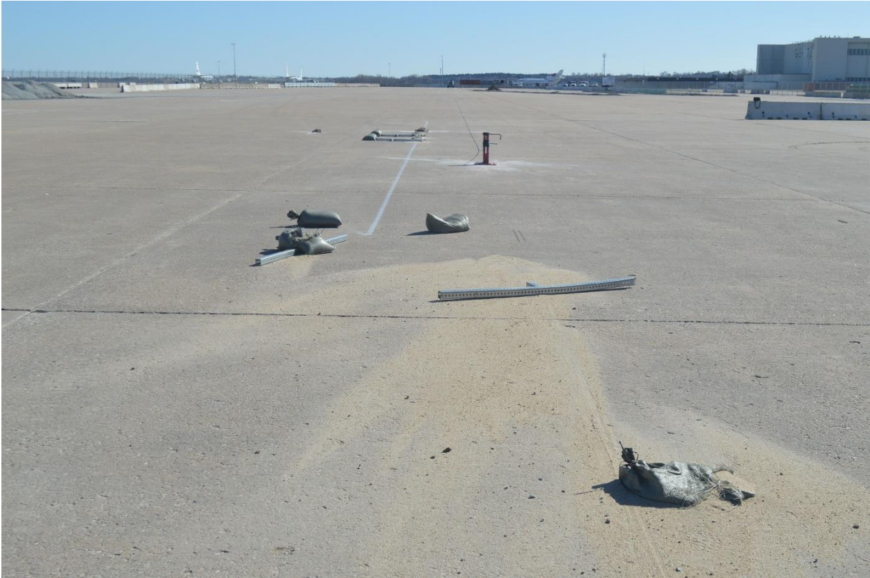
Figure 24. Overall System A and System B Damage, Test No. WZNP-2
