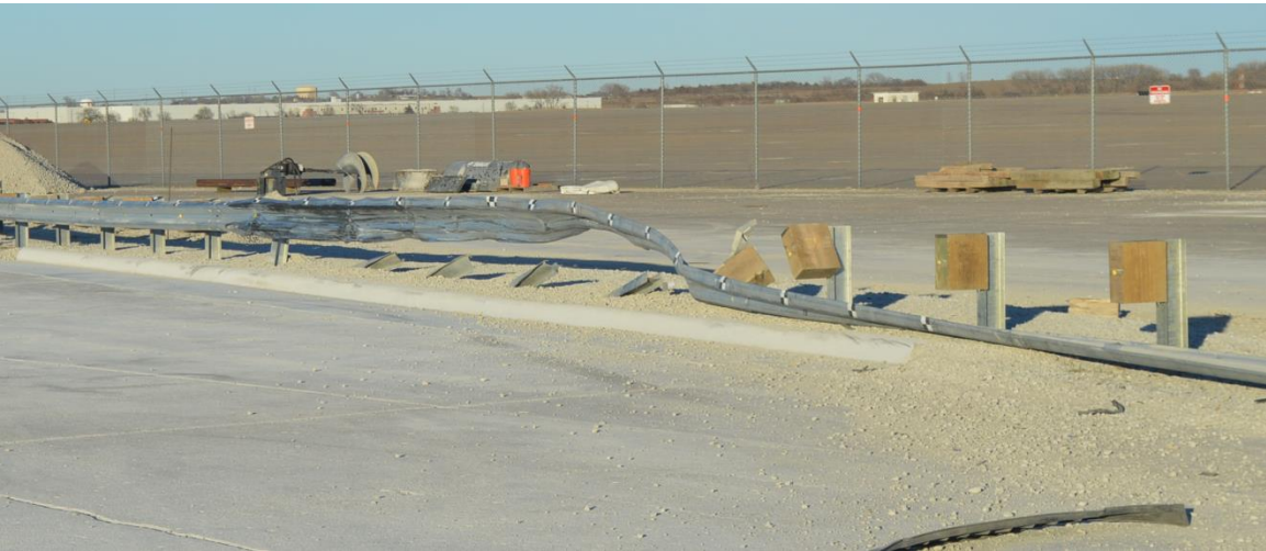
Figure 71. System Damage, Test No. MGSC-8
