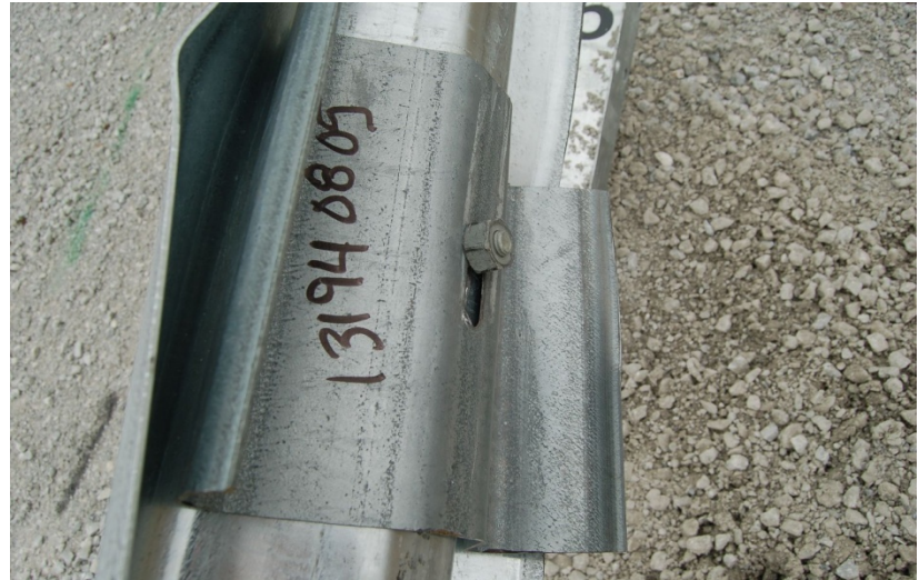
d. Backing Plate at Post No. 14
