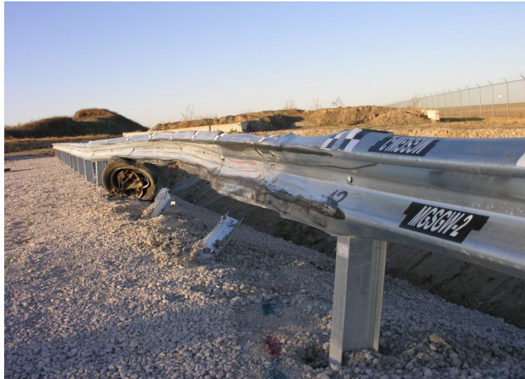
a. Impacted Rail
