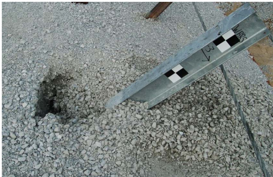
Figure 13. Photo. Typical Damage - 6-ft (1.8-m) Long, W6x8.5 (W152x12.6) Post at Breakpoint of 3H:1V Fill Slope.
