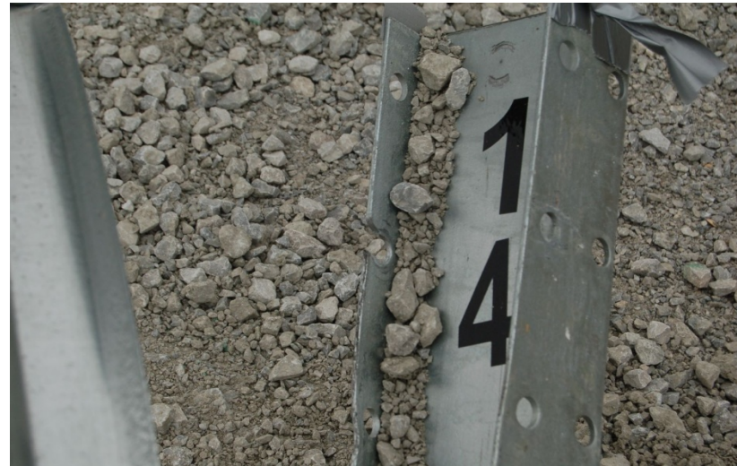
d. Post No. 14, Post Bolt Hole Tear
