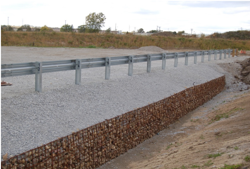
b. MGS on MSE Wall, Upstream Rear Quarter View
