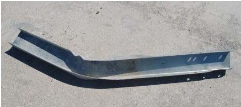
i. Post After Impact – Removed, Showing Deformation
