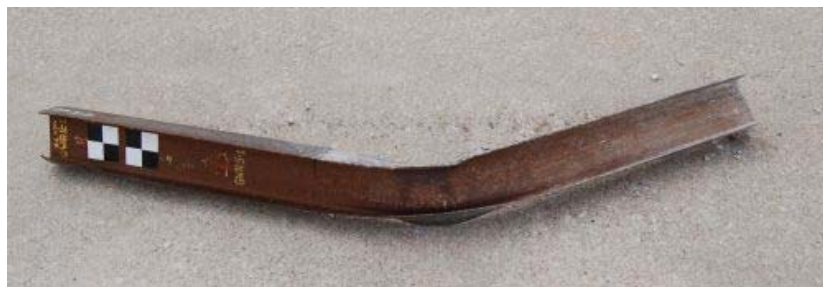
i. Post After Impact – Removed, Showing Deformation
