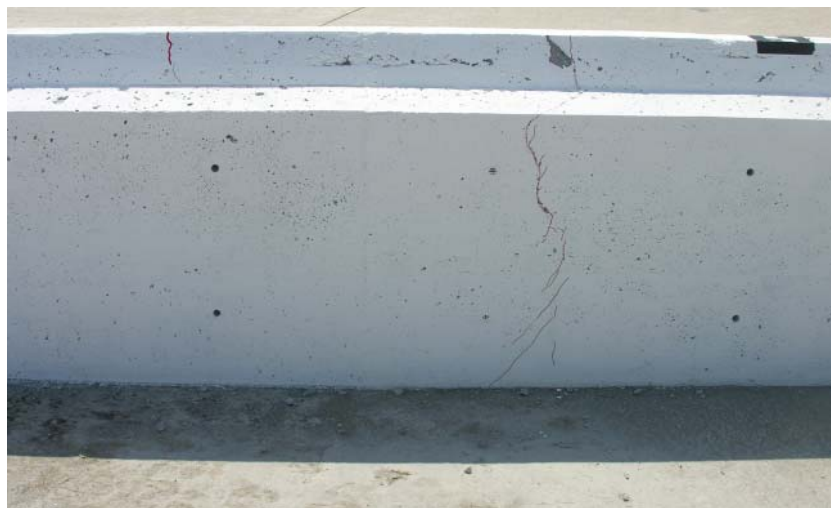
Figure 74. Barrier Cracks Upstream of Impact, Test TL5CMB-2
