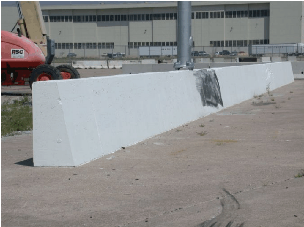
Figure 50. System Damage, Test No. ZOI-2
