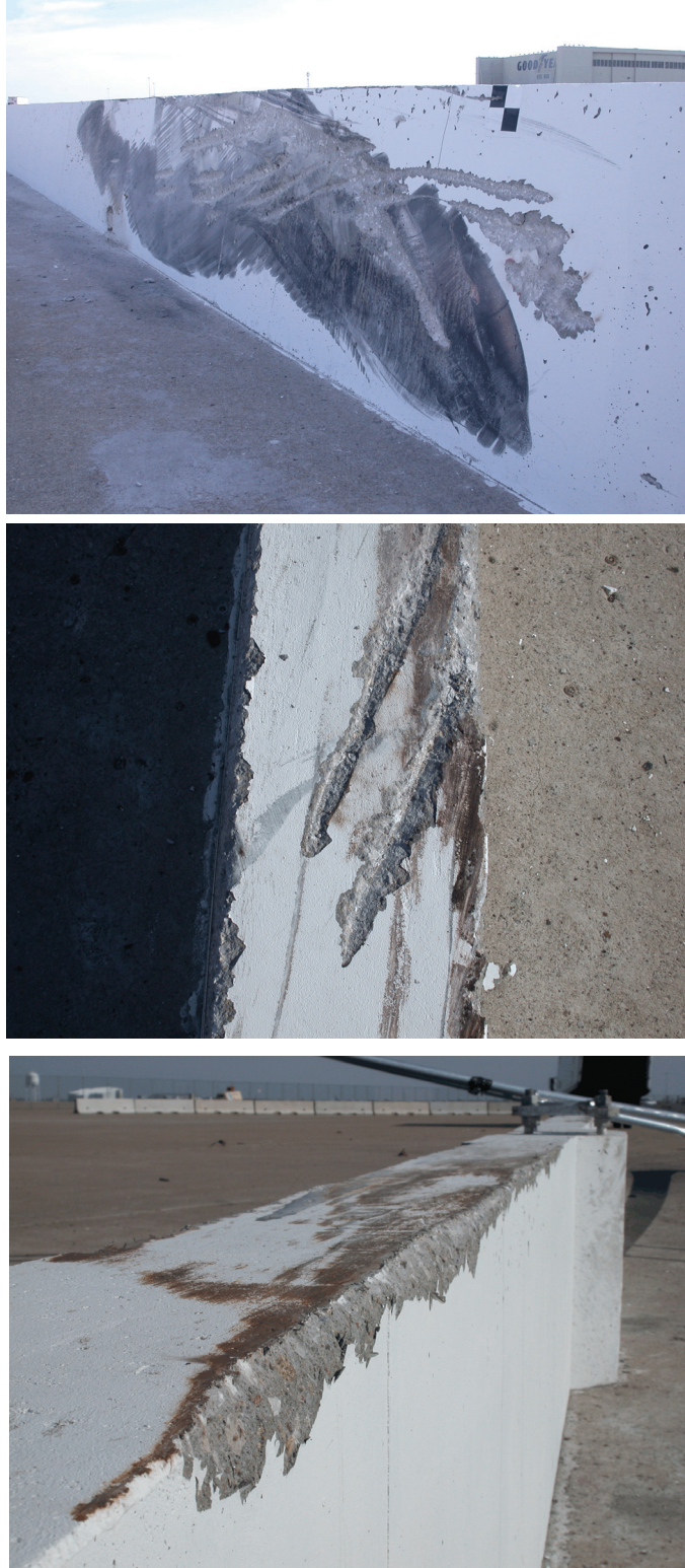
Figure 36. System Damage, Test No. ZOI-1
