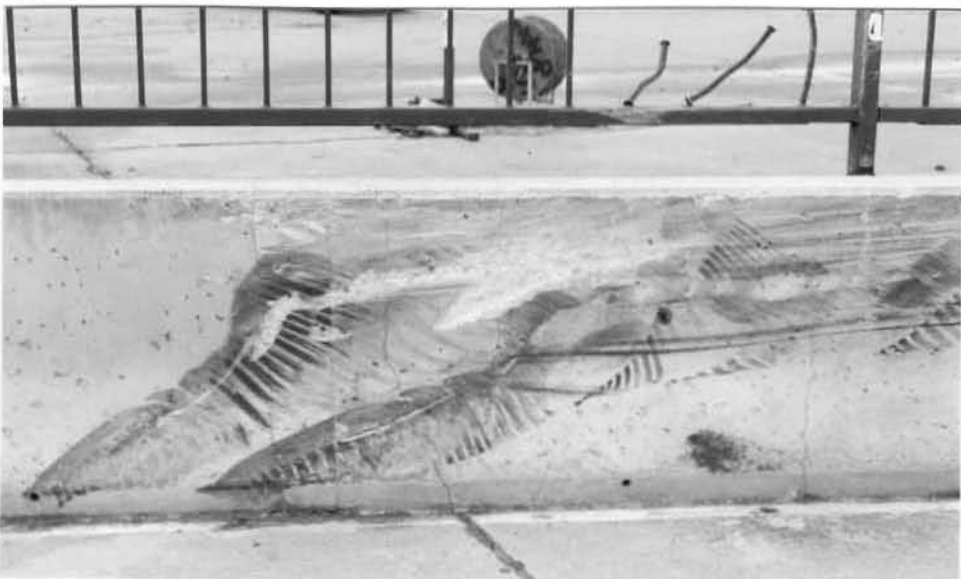
Figure 24. Barrier Damage, Test MNPD-1
