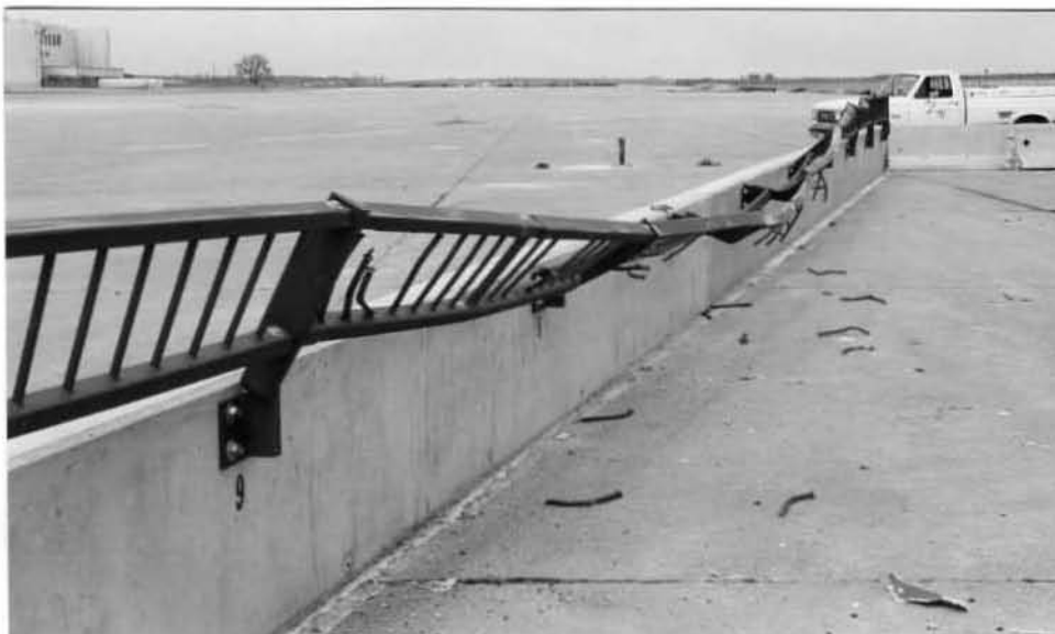
Figure 34. Barrier Damage, Test MNPD-2
