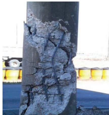
Column shear failures
