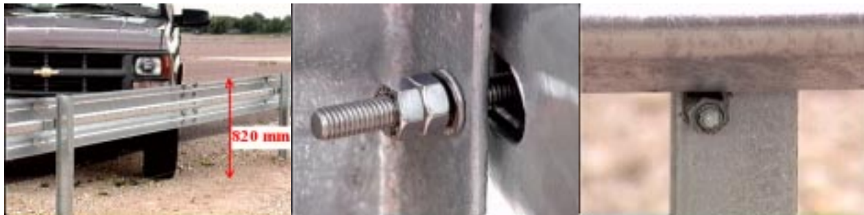
(A) Midspan splices, rail height and backup plates. (B) Improved connection. (C) Rail support bolt.
