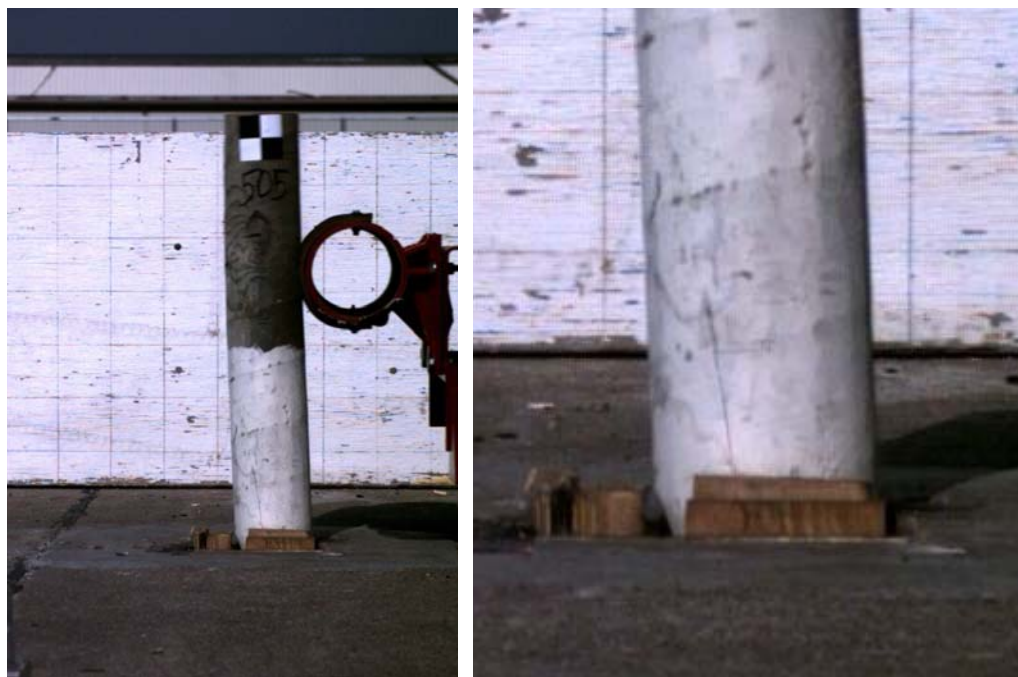
Figure 12. Post Bending Prior to Fracture - Frame 107
