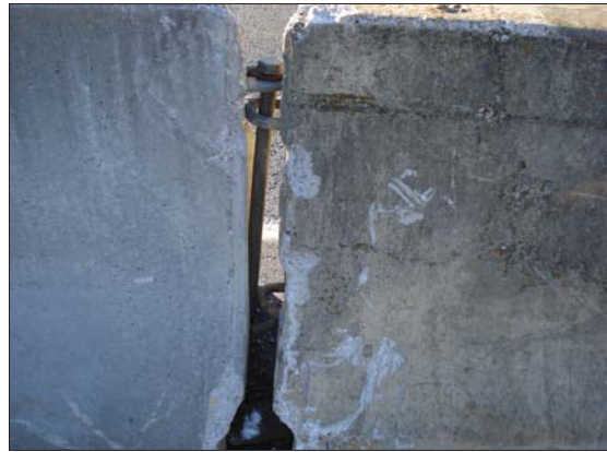
X Not Bolted at Bottom
