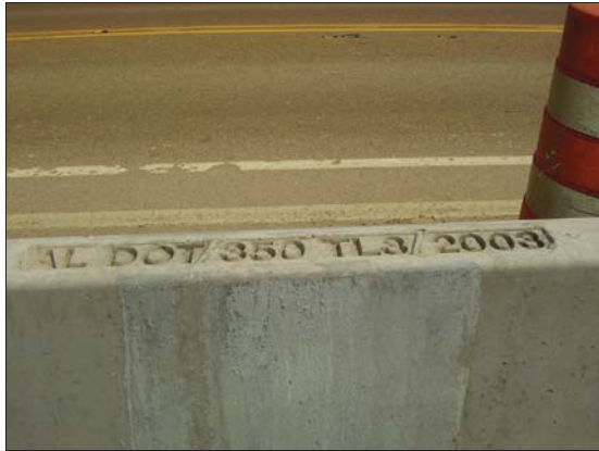
✓ Info Properly Embossed On Top of Rail
