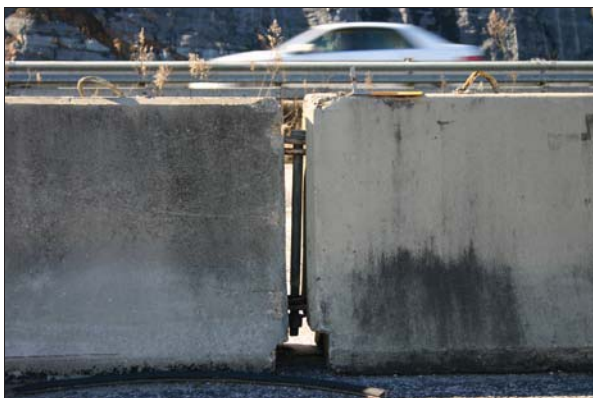
✓ Good Condition (Bolt and Loop Type)
