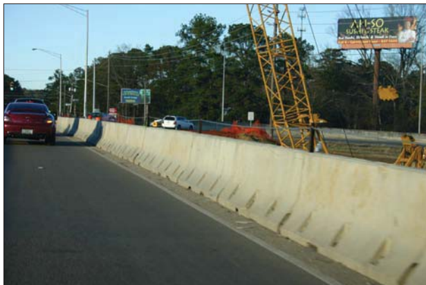
X No Reflectors On Top of Rail
