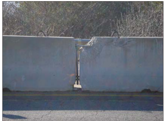
X Physical Damage
