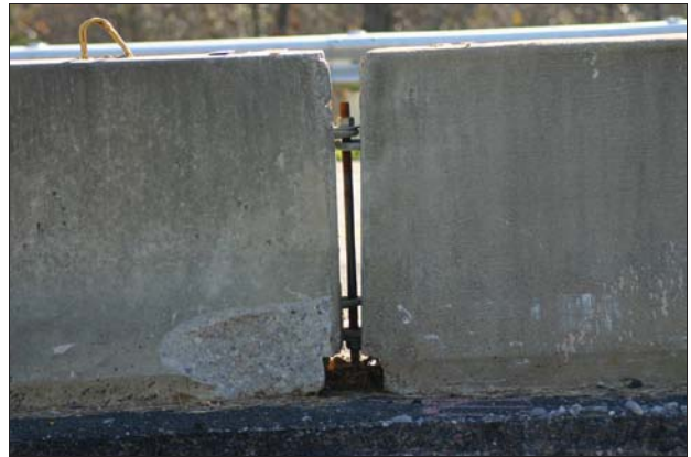
X Bolt Too Small (Minimum Diameter 1 1/4" Required)
