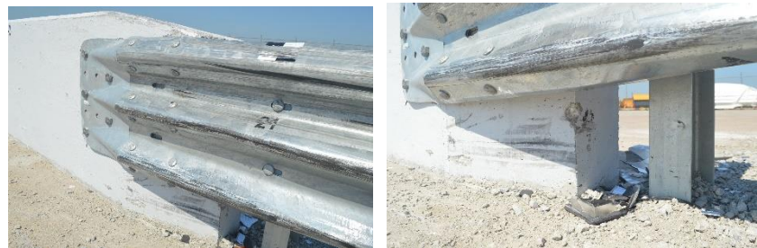
(c) AGT and Buttruss Damage
