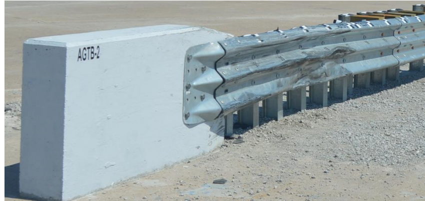
(b) System Damage
