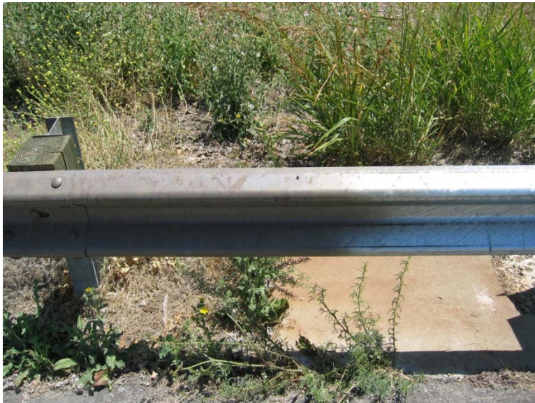
Figure 34 - Comparison of Staining Product and Galvanized Steel Guardrail
