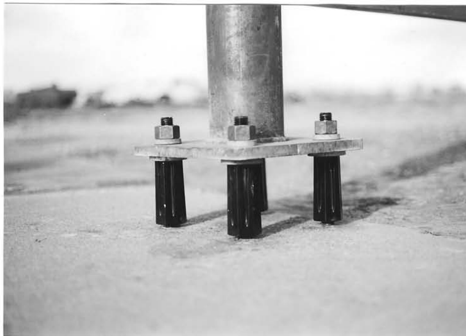
Figure 10. Installed Breakaway Couplings
