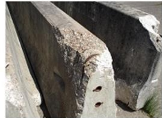
(f) A large spalled area with exposed reinforcing bars
