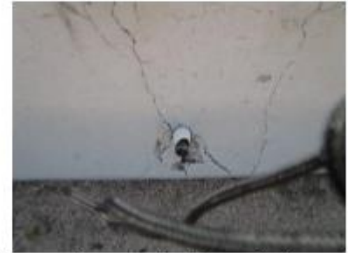
(f) A crack extends through the anchor hole.
