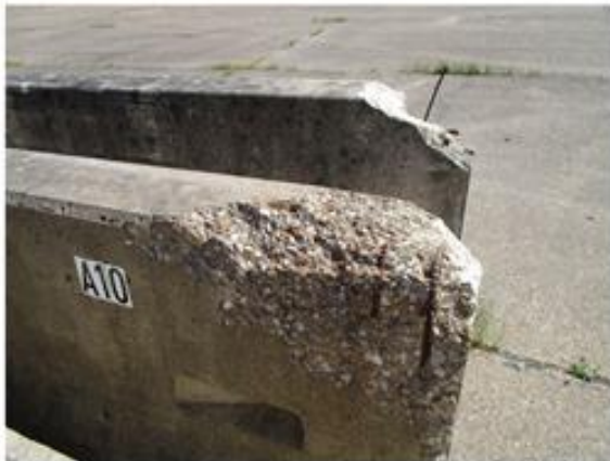
(c) Exposed reinforcing steel
