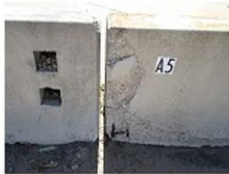
(e) Large spalled area
