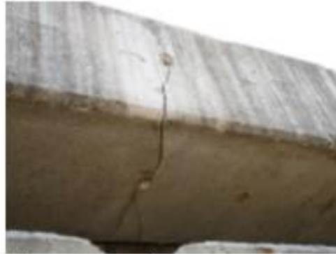
(e) Large crack
