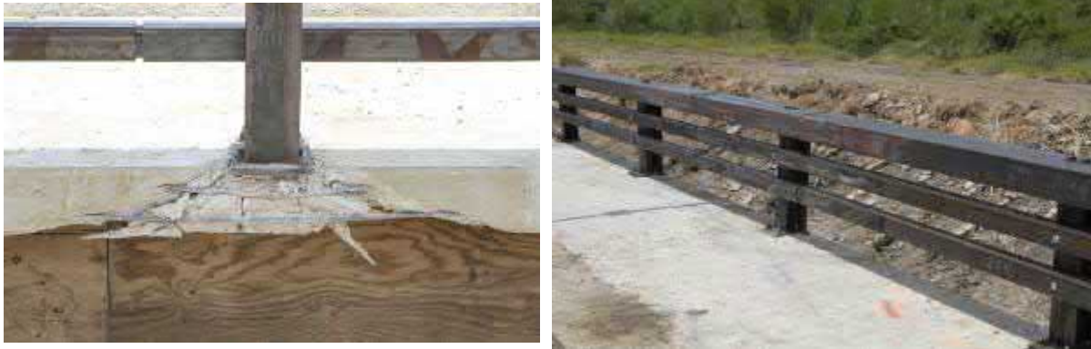
Figure 3.27 Damage to TxDOT T131 Bridge Rail (18) .
