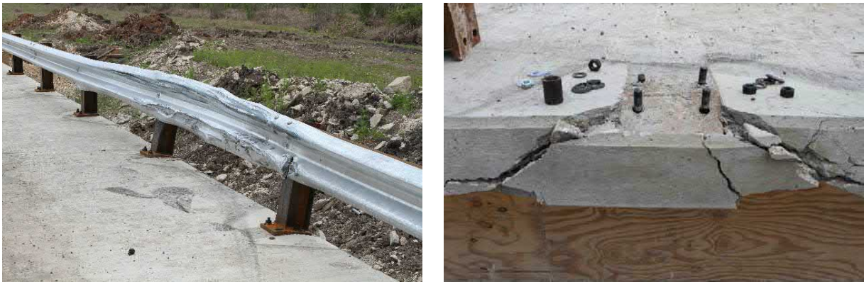
Figure 3.26 Damage to TxDOT T101 Bridge Rail (17) .
