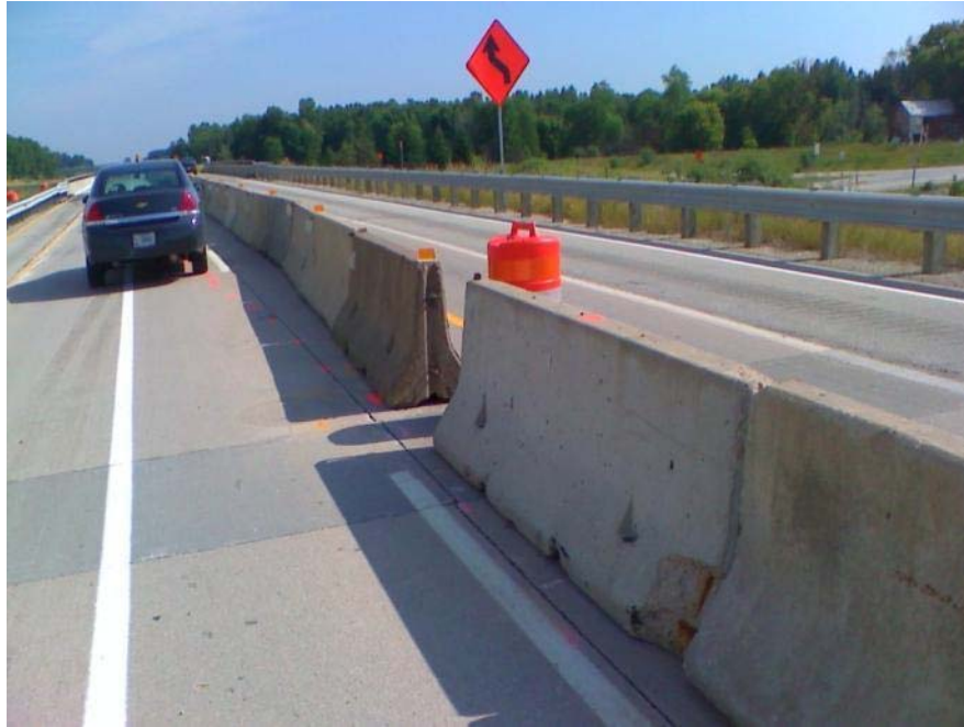
Figure 20 Gap in Barrier
