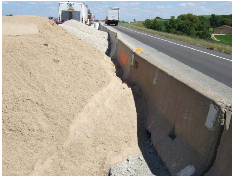
Figure 21 Insufficient Clearance Behind Temporary Barrier
