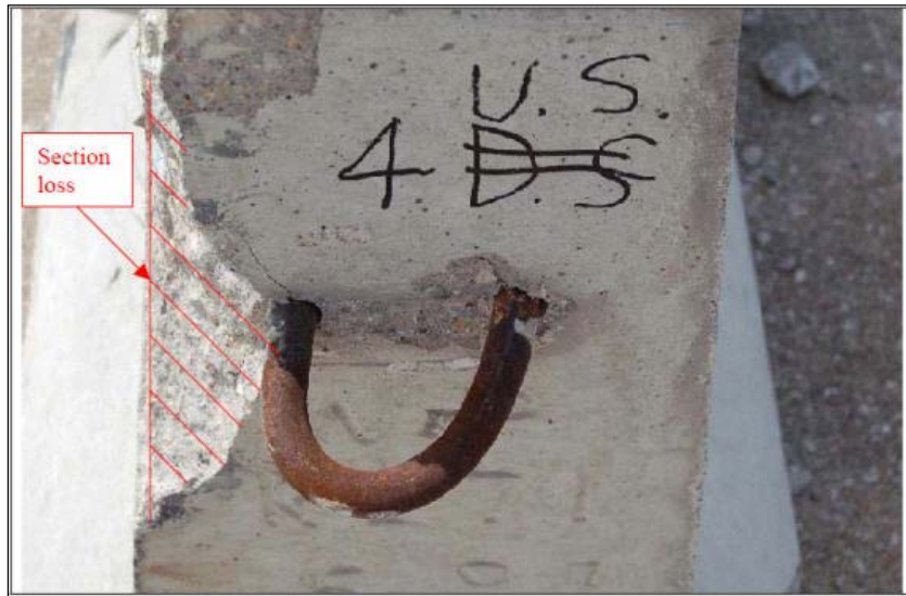
Figure 5 Loop Out of Alignment
