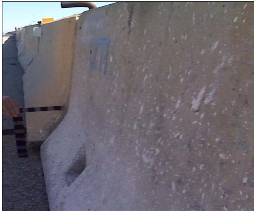
Figure 16 Potential Snag Point Caused by Different Barrier Styles Not Matching Up
