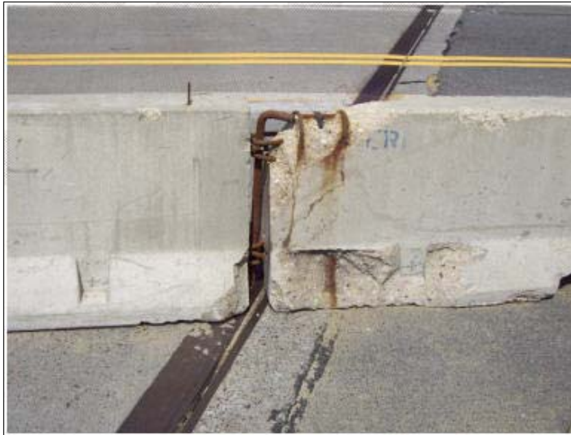
Figure 7 Exposed Steel and Section Loss Near End Section
