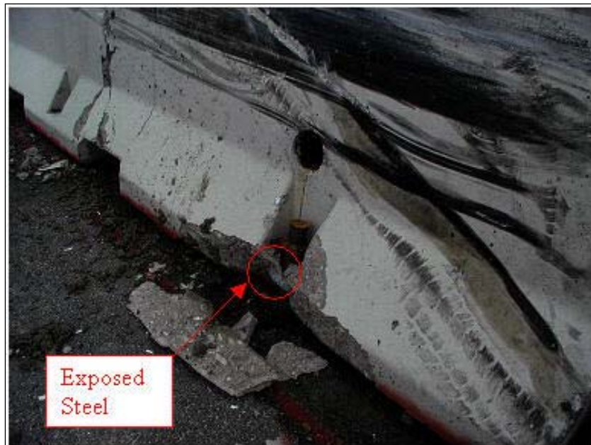
Figure 8 Anchor Hole Damage
