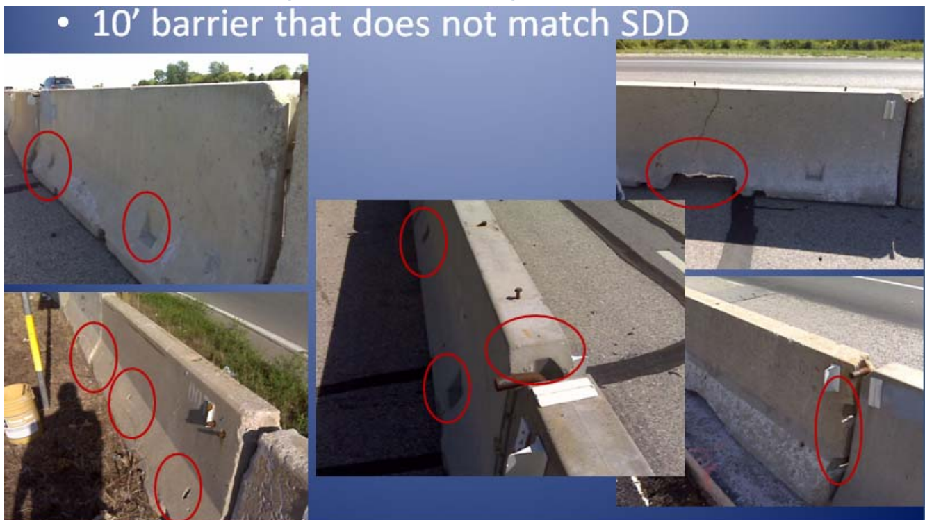
Figure 23 Barrier Not Matching Standard Details
