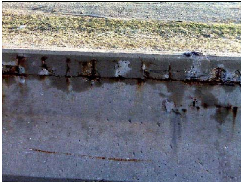
Figure 10 Exposed Steel Reinforcement
