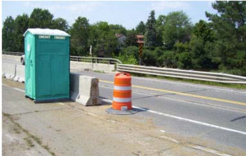
Figure 19 Improper Termination of Barrier and Object within Deflection Distance
