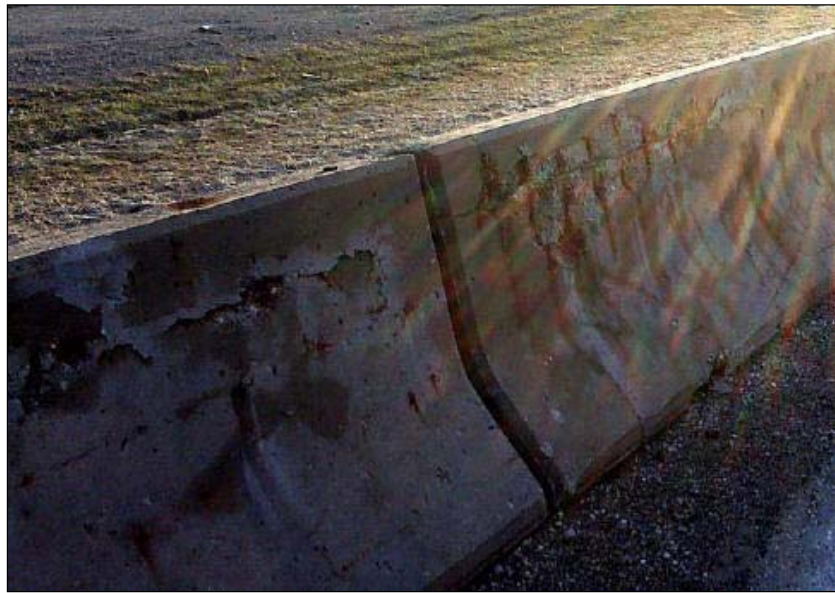
Figure 11 Exposed Steel Reinforcement
