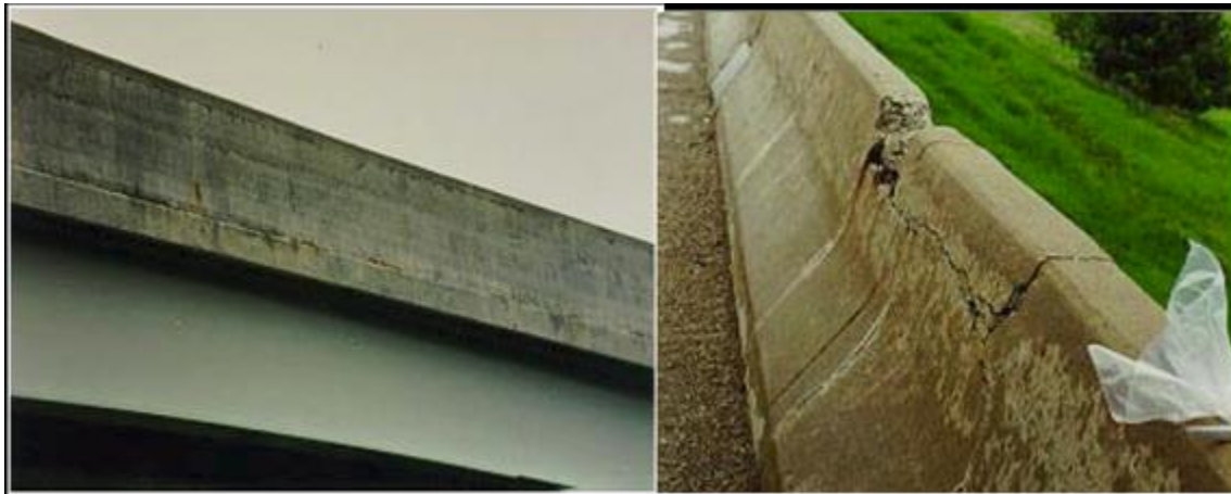
Figure 10: Typical advanced deterioration of horizontal cracks (Staton and Knauff, 2007)
