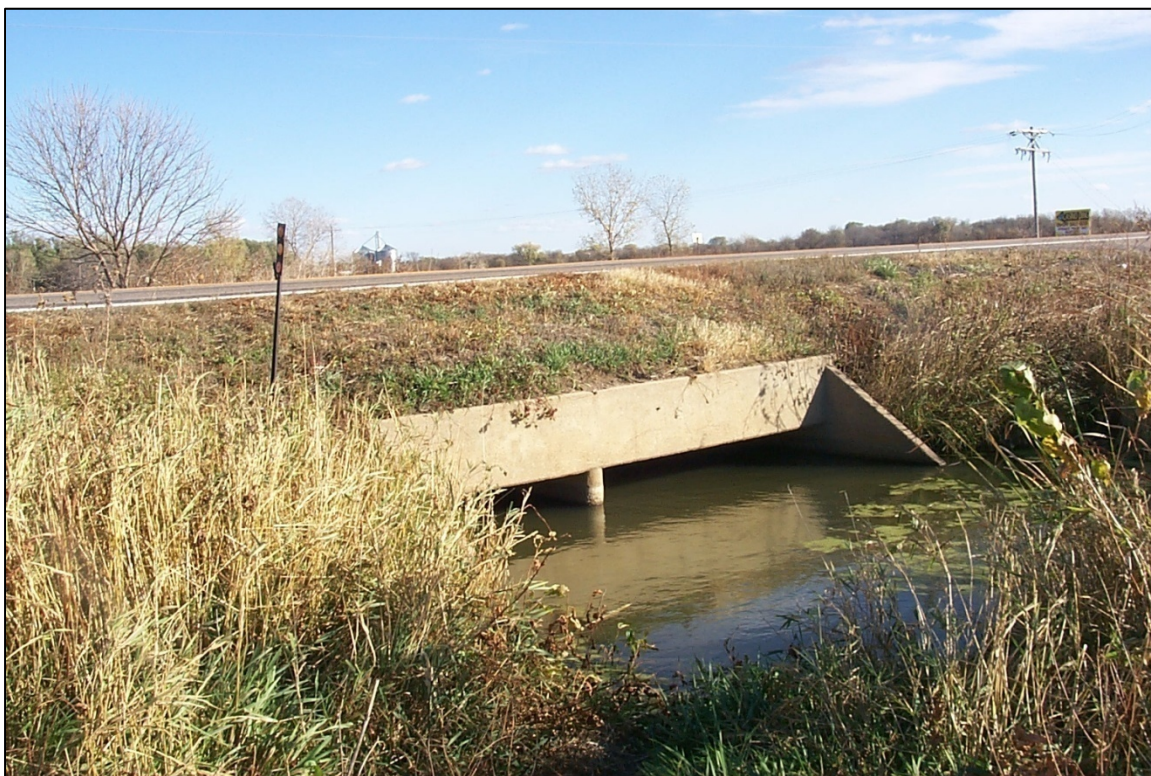
Figure 6. Unprotected roadside culvert
