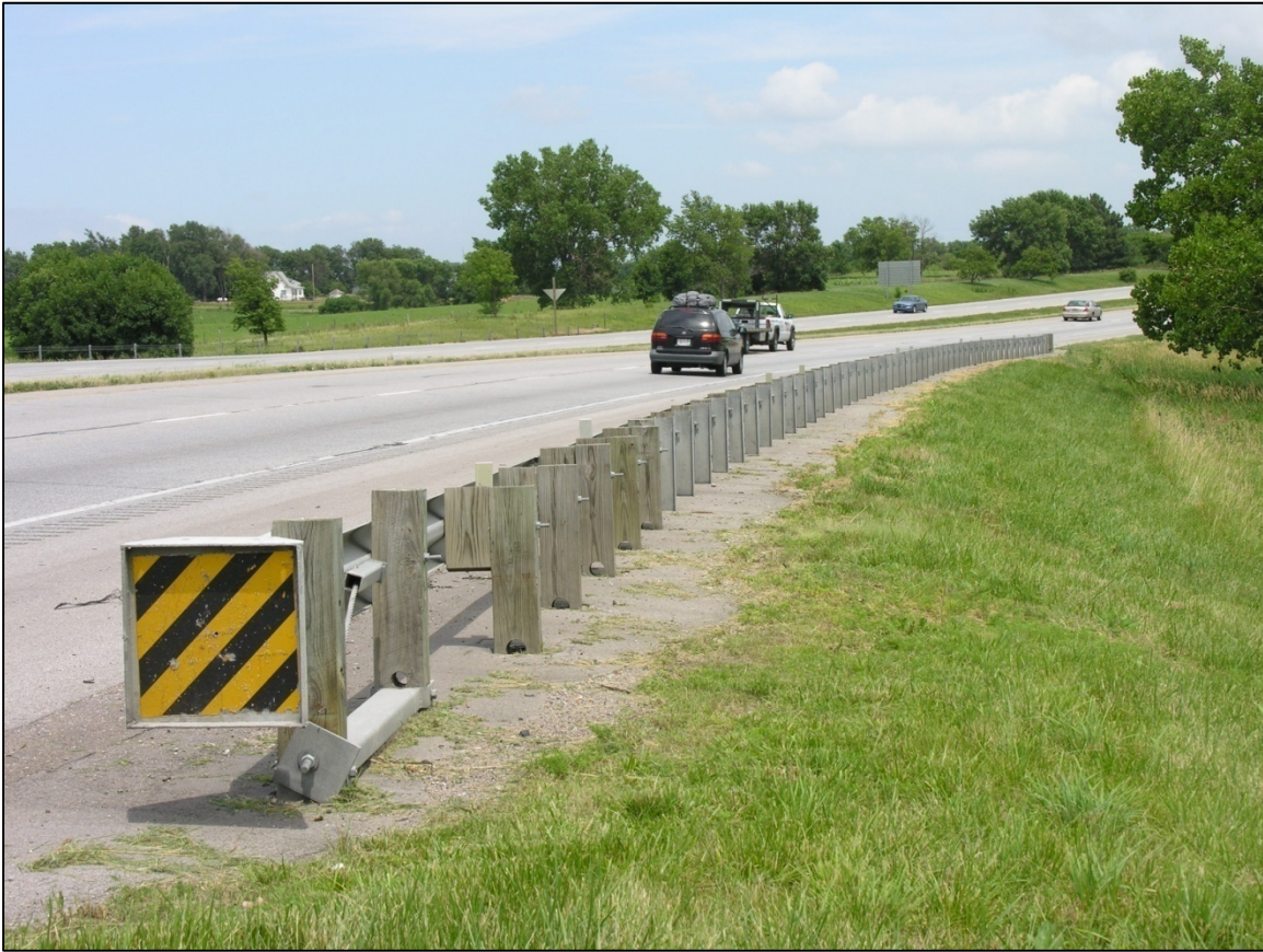
Figure 21. Upstream side guardrail end-terminal
