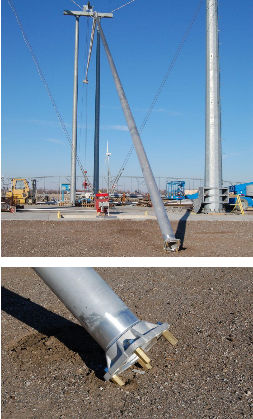
Figure 69. System Damage, Test No. BBC-7
