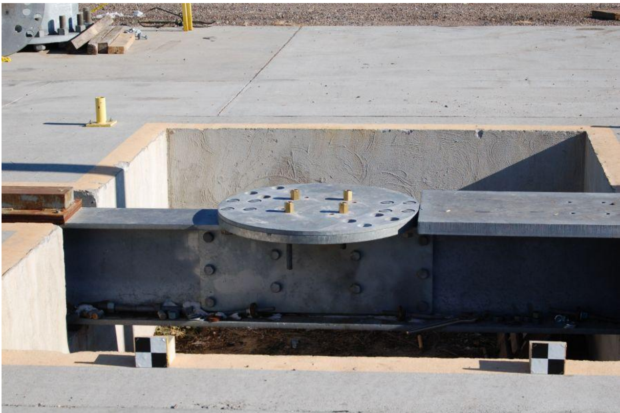
Figure 64. System Damage, Test No. BBC-6
