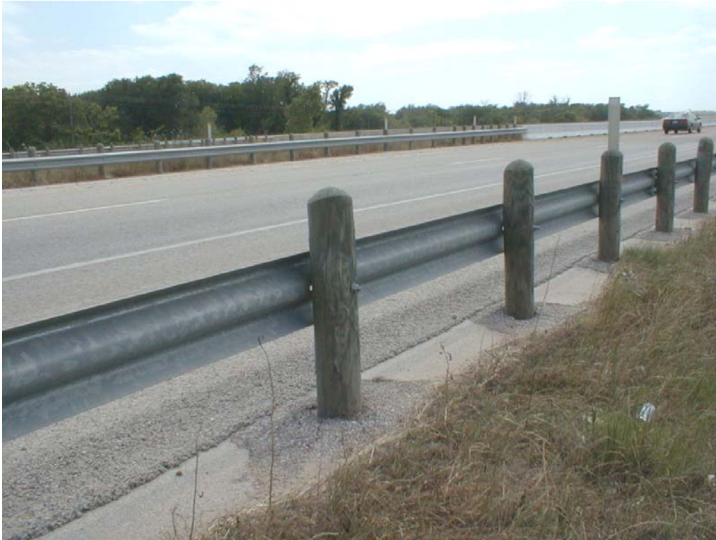
Figure 2. Wood Post Guardrail System with Asphalt Mow Strip.
