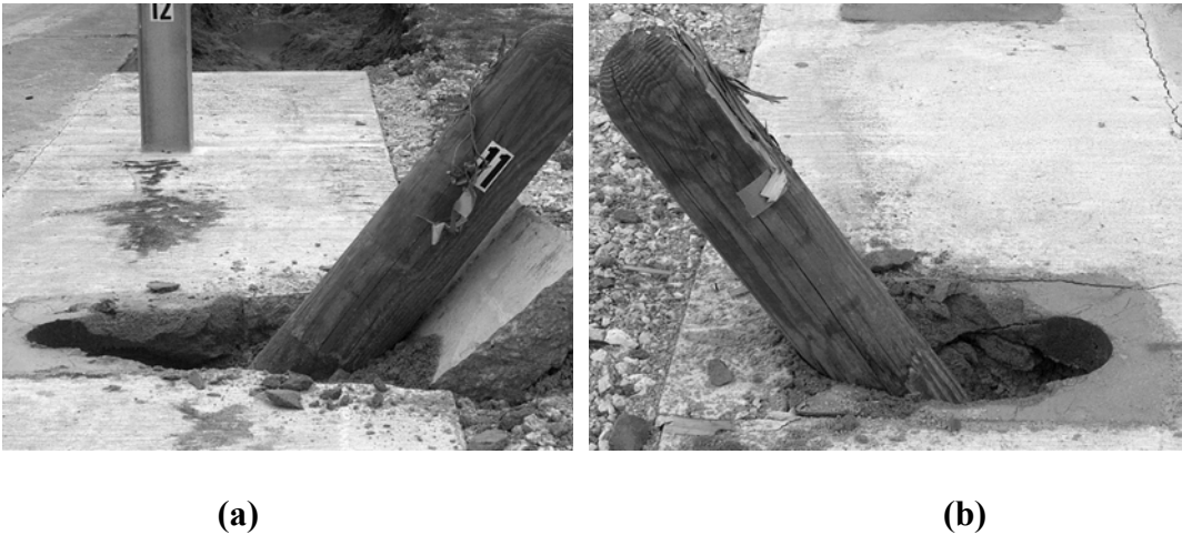
Figure 22. Wood Posts in Concrete Mow Strip with Grout-filled Leave-out: (a) Square Leave-out; (b) Rectangular Leave-out.
