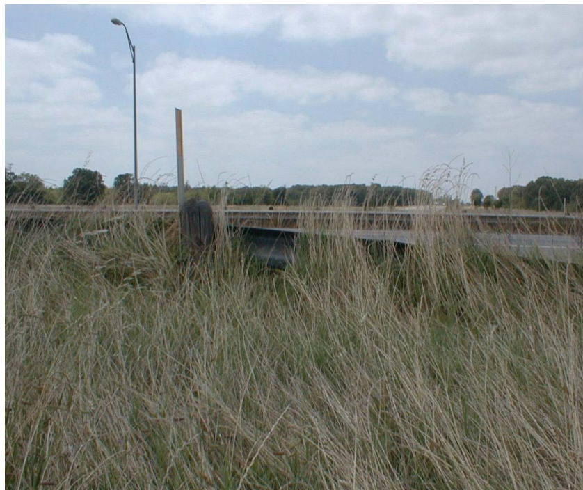
Figure 1. Guardrail Installation Overgrown with Vegetation.
