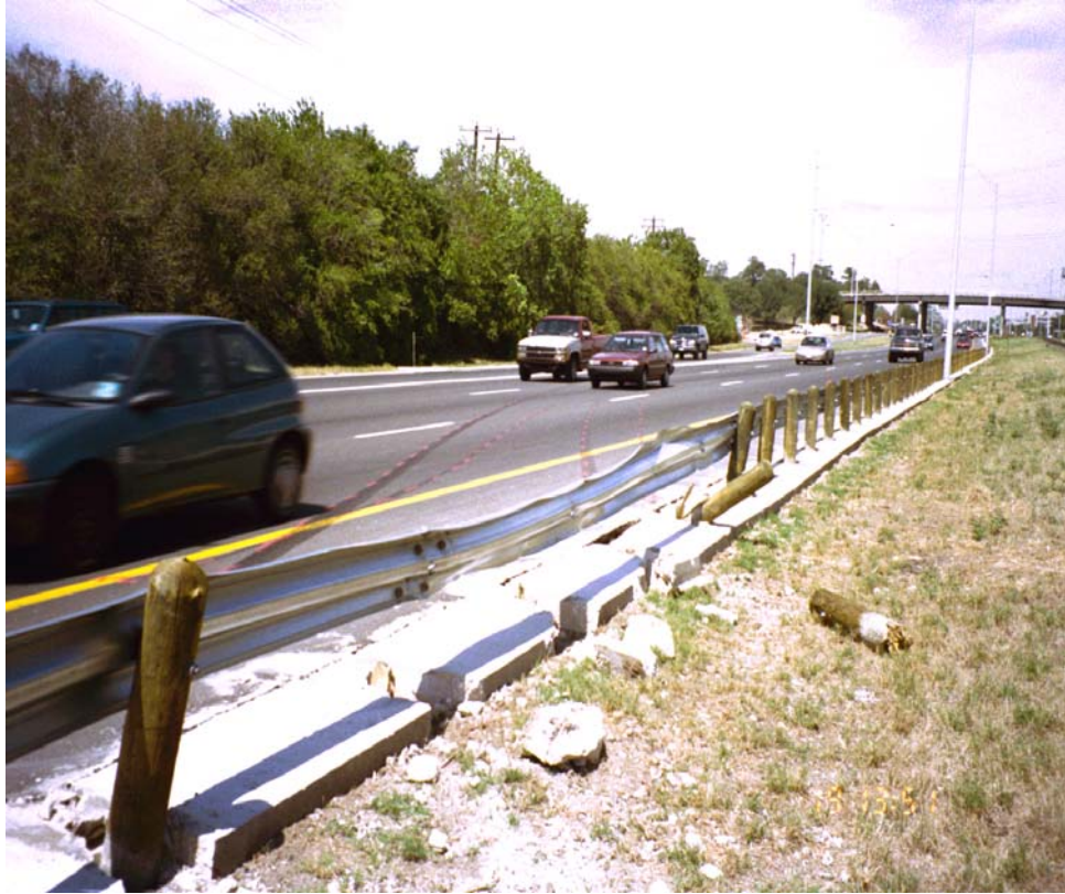
Figure 4. Mow Strip Guardrail System after Impact.
