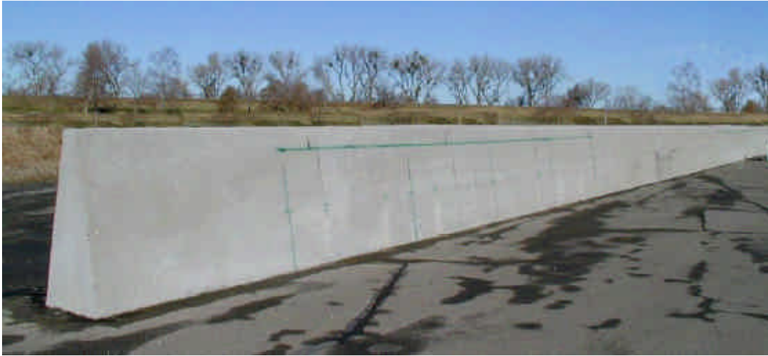
Figure 2-1 Existing Type 60G barrier
