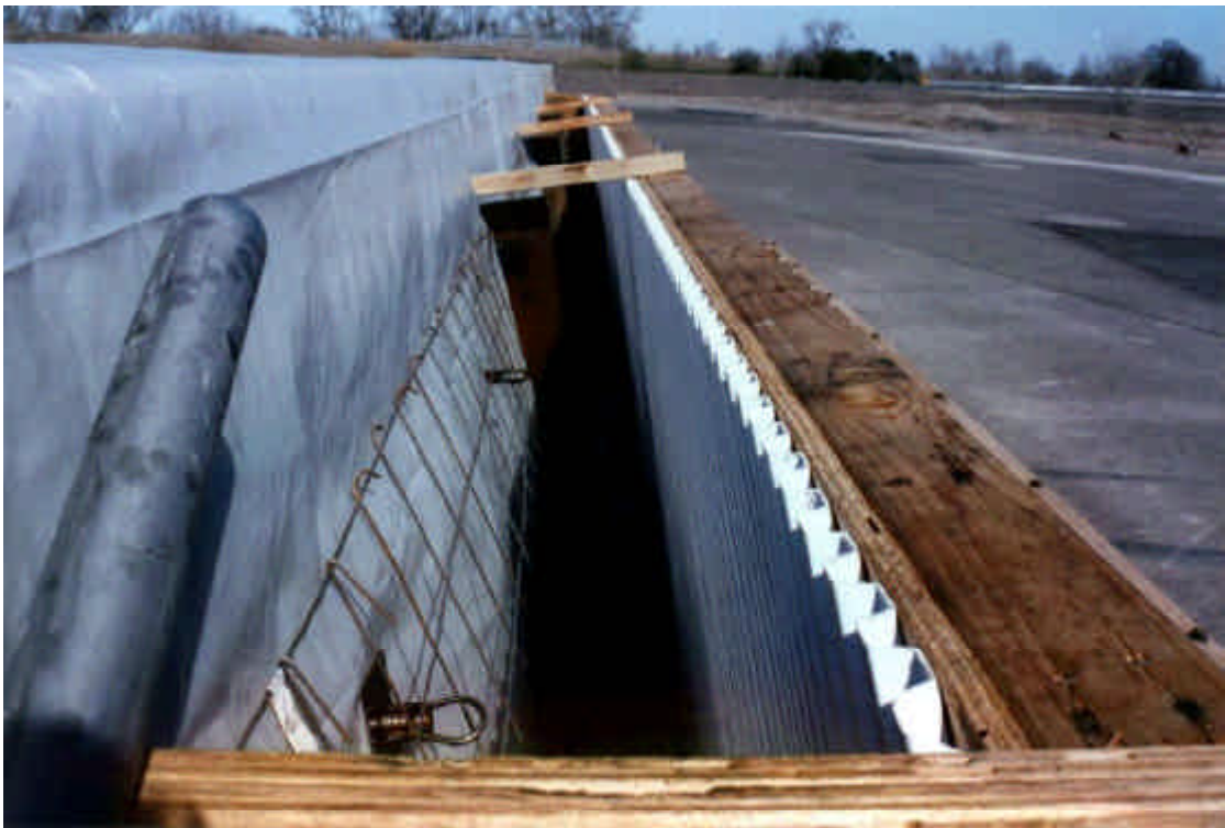
Figure 2-2. Formwork ready for concrete placement (note the plastic sheeting and ferrule loop inserts)
