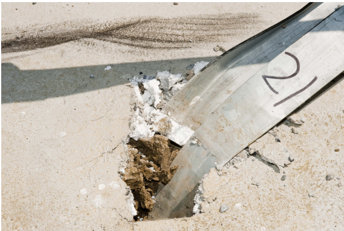
Figure 2-41 – Close-up of Post 21 after Test 659
