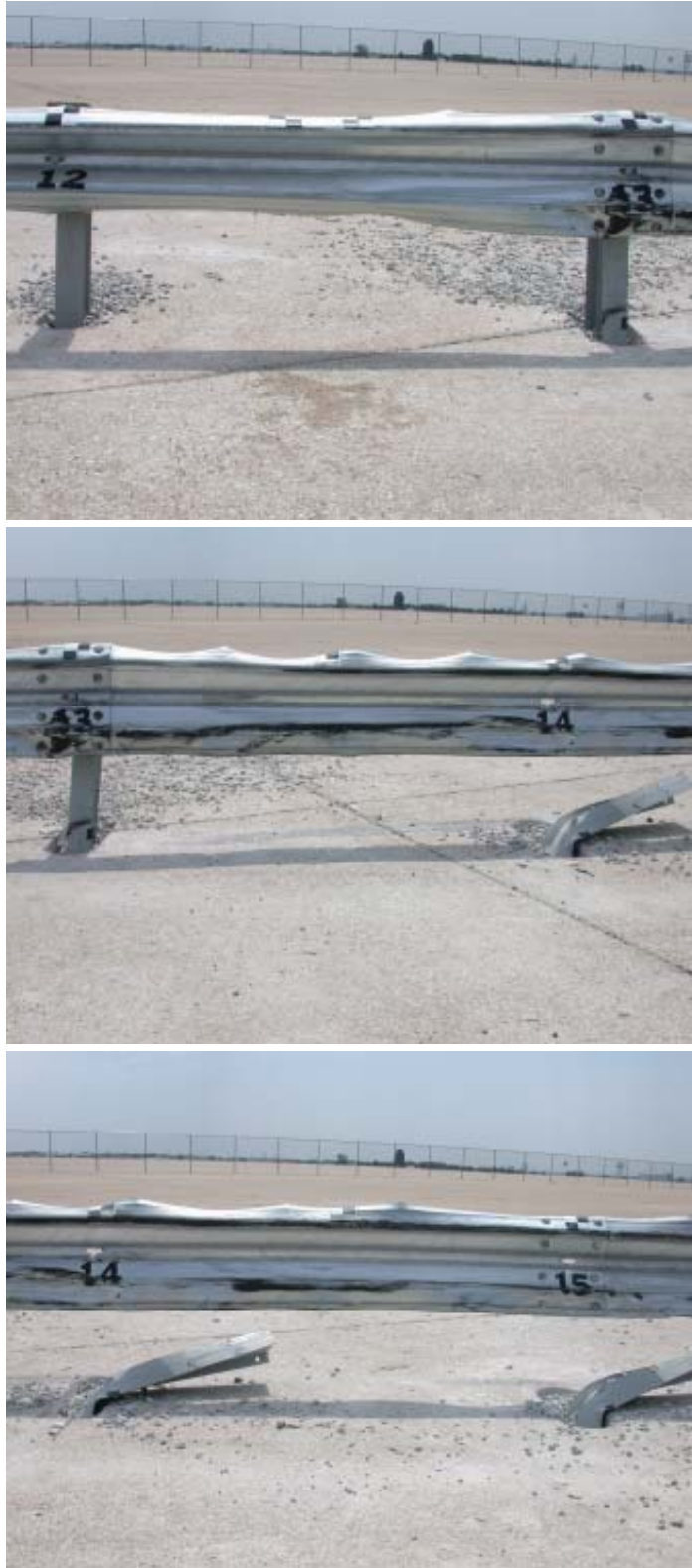
Figure 46. W-beam Guardrail System Damage, Test PR-1
