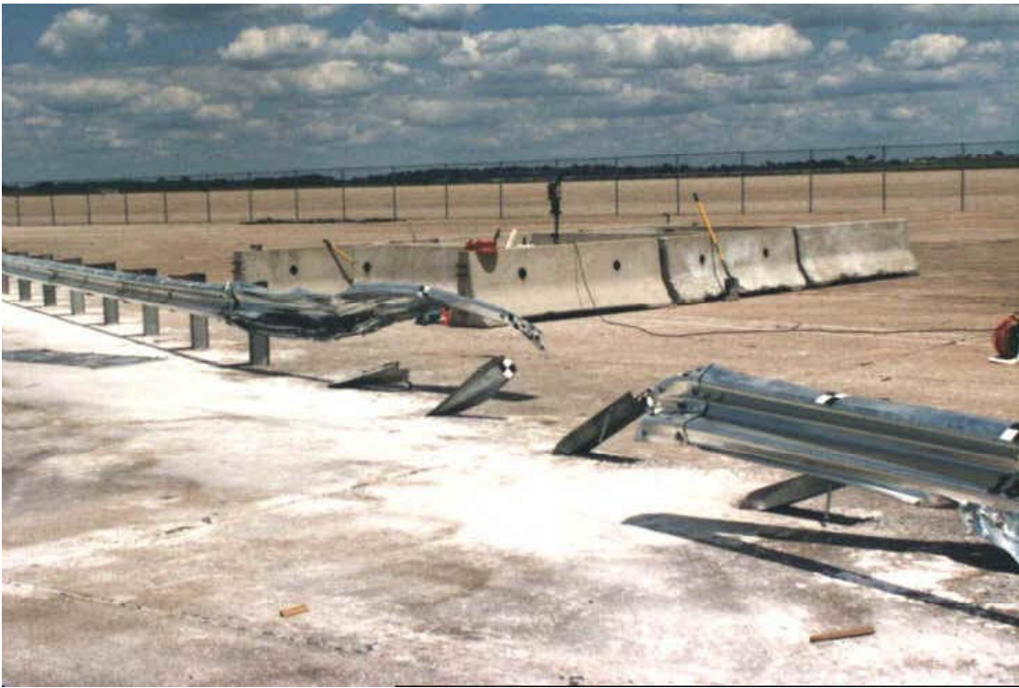
Figure 2. W-beam Guardrail System Damage, Test RP-1
