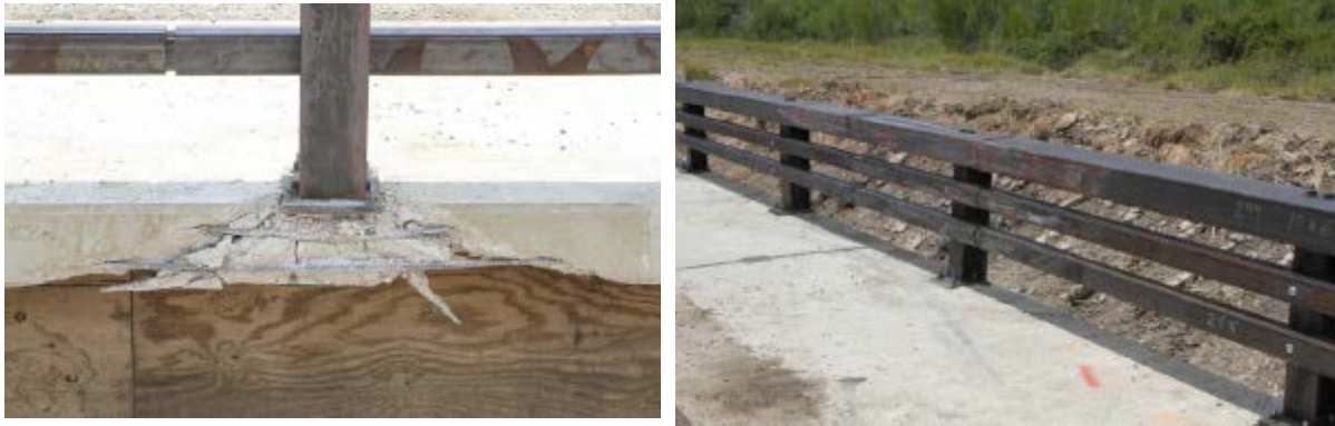
Figure 3.27 Damage to TxDOT T131 Bridge Rail (18) .
