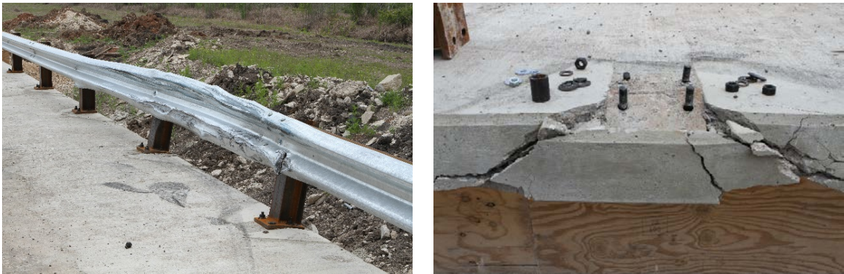
Figure 3.26 Damage to TxDOT T101 Bridge Rail (17) .
