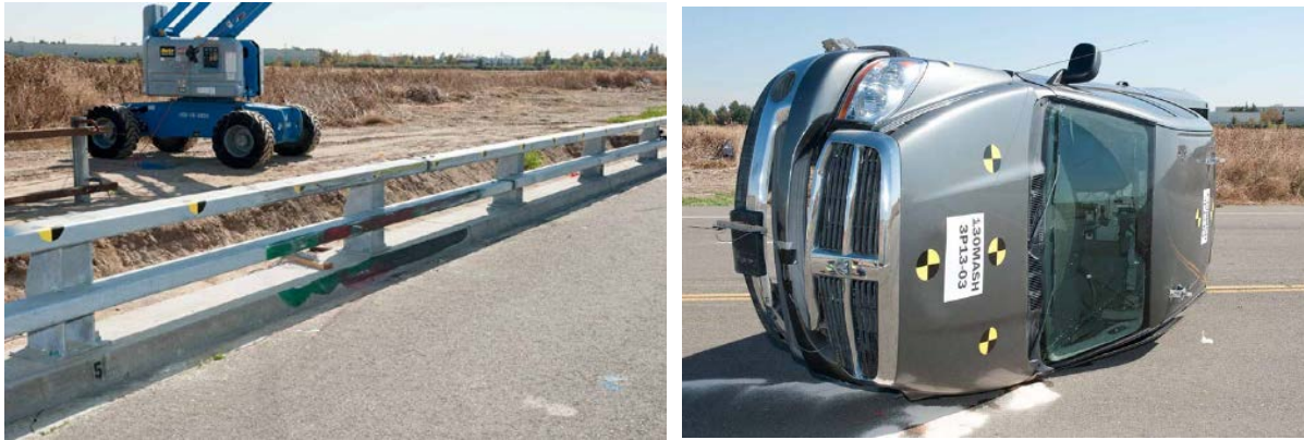
Figure 3.32 Damage to Barrier and Vehicle for ST-10 Bridge Rail (19) .
