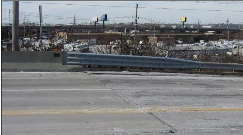
Figure 13. Reinforced concrete bridge railing and metal transition railing for Bridge Number 15558X.
